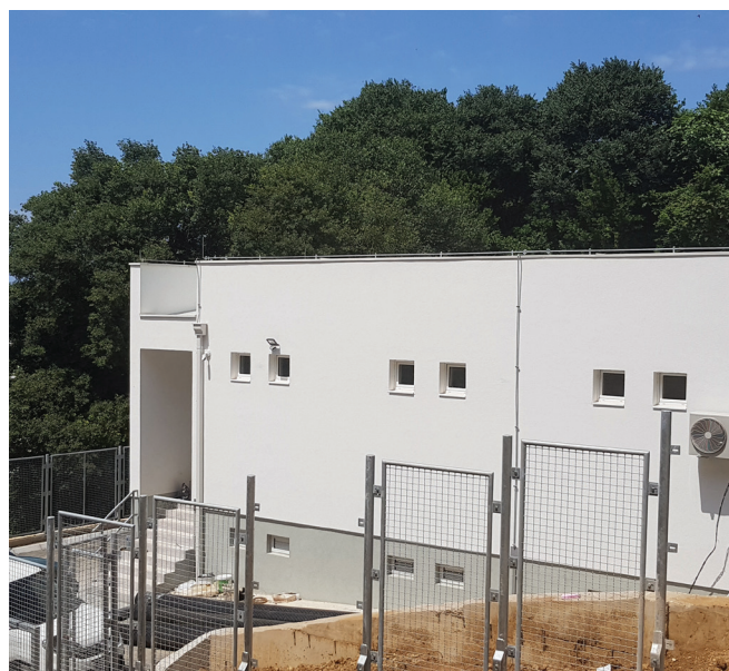
TS 35/10kV “Novi Ulcinj”
